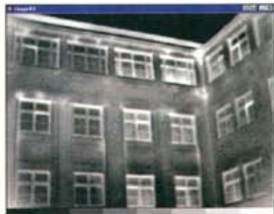
Figure 3: Infrared thermography reveals hot spots that are usually air leaks.
